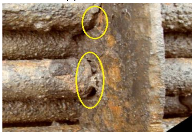
Figure 3. Corrosion of connections between pipes, piping network and barriers
